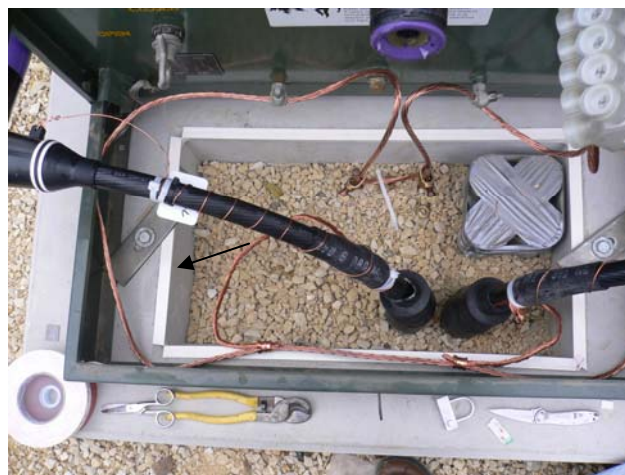
Figure 1. Pad mounted electrical transformer box containing ARINIX permethrin impregnated nylon plastic strips.
